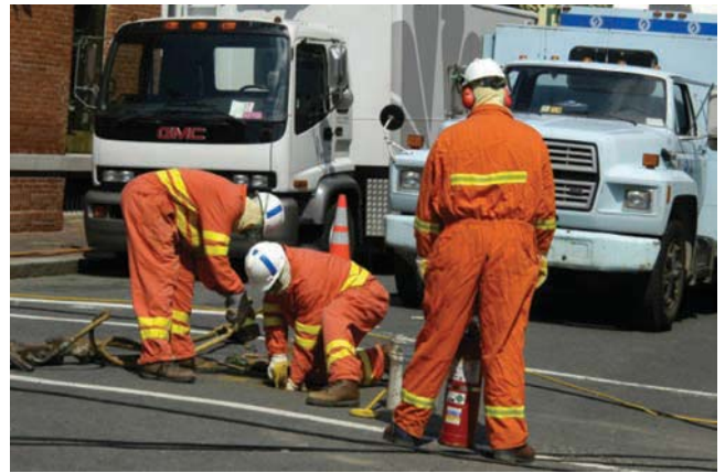
Gas company employees repairing a utility line on a road in Alexandria, Virginia
